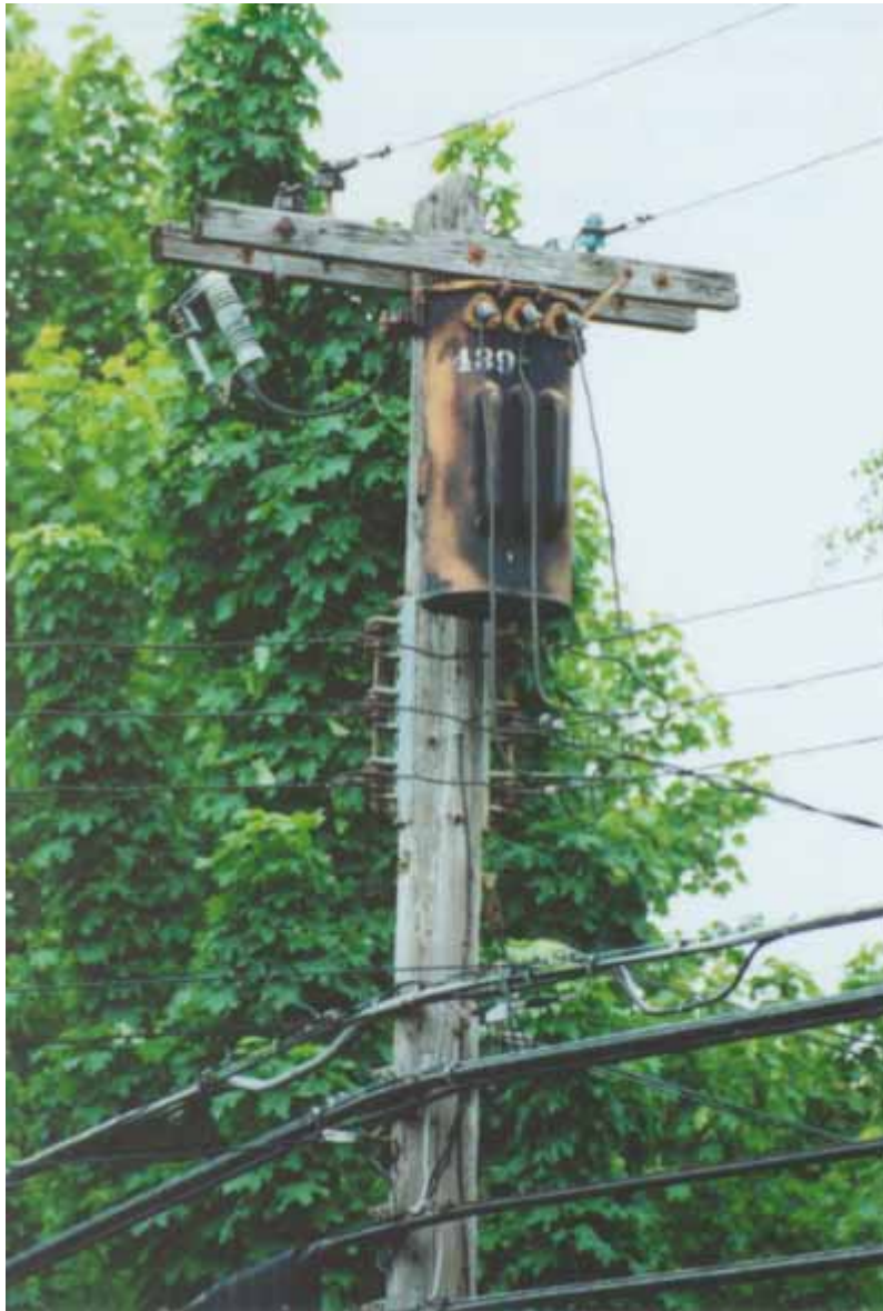
Transformer with paint showing evidence of deterioration and old-style connectors
